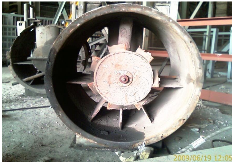
Fig 1: The Impeller with broken blades
